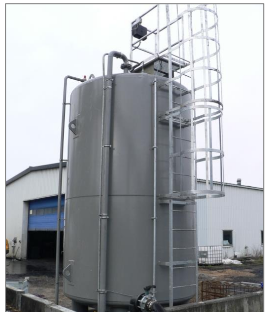
20 m 3 tank diameter Ø 2500 mm. With ladder and platform on top of tank, fill point to ground level, leak detection system etc.
