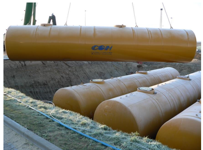
4 x 100 m 3 double skinned tanks
