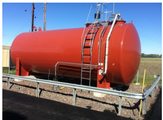
50 m 3 tank diameter 2900 mm. Ladder, platform and railing on top of tank. Fill point to ground level.
