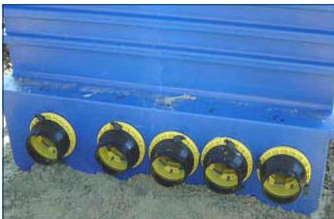
"Easy Fit" pipe entry fittings installed in a dispenser sump. Four secondary contained suction lines and one vapour recovery line are to be connected.
